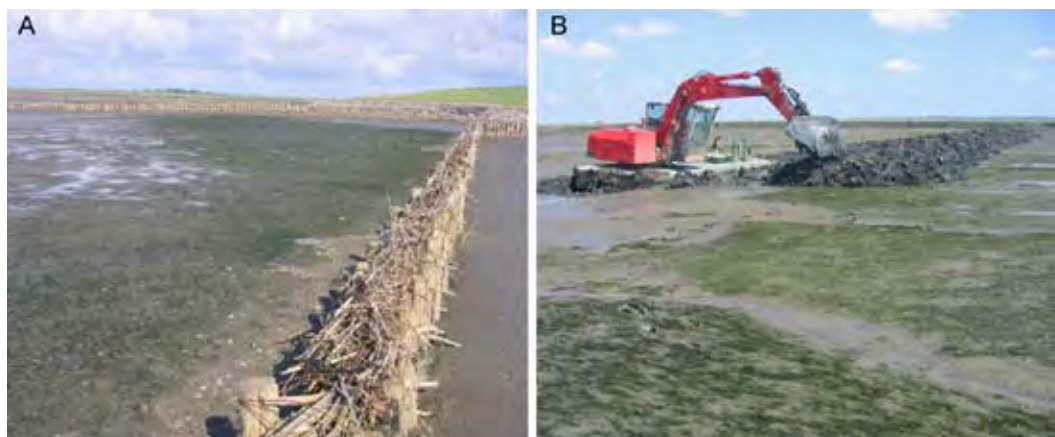
Figure 5: Depending on the hydrodynamic regime, seagrass can benefit from brushwood groins when they cause stable sediment conditions (A; south of Eiderstedt peninsula). However, severe damage can be done to a seagrass bed when drainage ditches are dug as happened at Hamburger Hallig (B) (Photos: T. Dolch, August 2008).
